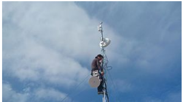
Installation of a "supernode" of fguifi.net 's community network in Tarragona
