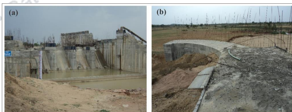
Fig. 5.26 (a) An spillway under construction for a 16m high earth dam, also see the stilling basin. (b) Sides of spillway to act as abutment over which earth will rest.
